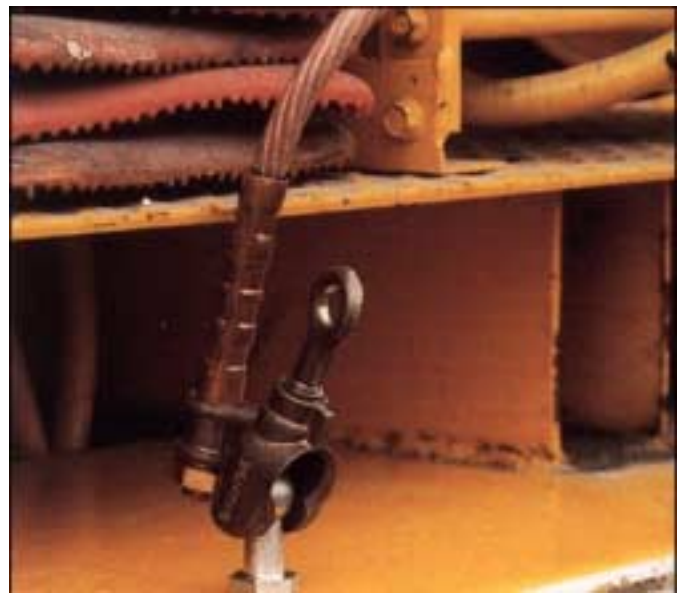
Figure 3 - Ball and Socket Grounding Connection
